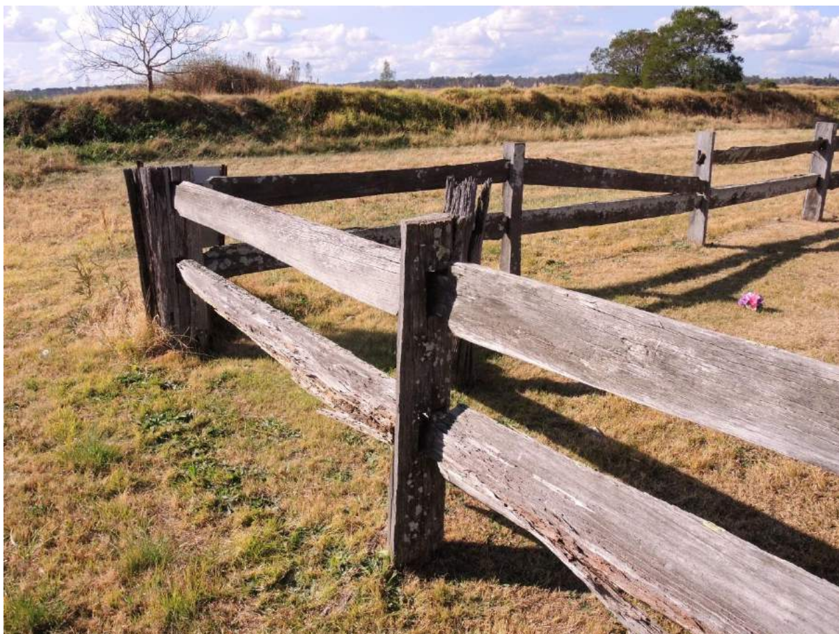
Figure 10: A relatively intact section of the perimeter fence, with a post from the earlier fence inside, at the northwest corner of the cemetery. The replacement fence should be of identical style and construction and made with timber treated to resist termite attack. (Source: Chris Betteridge, 2014)
