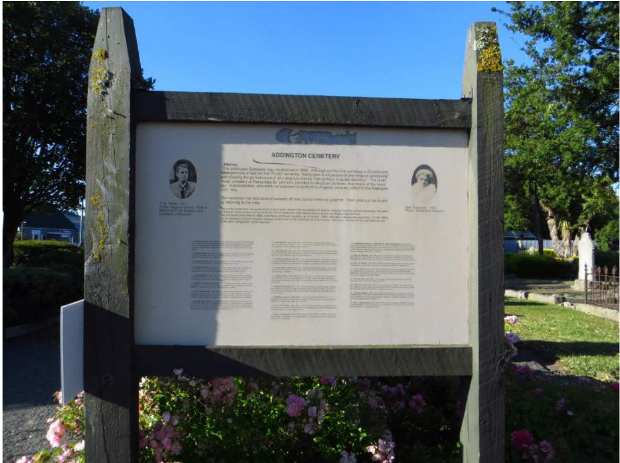
Figure 12: The sign at the entrance to Addington Cemetery in Christchurch, New Zealand, provides information about the history of the cemetery. Undressed, unpainted timber framing and supporting posts have allowed cracking and biological growth. (Source: Chris Betteridge, 2014)
